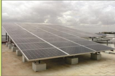
REVA Administrative Block, Bangalore IGBC Platinum
