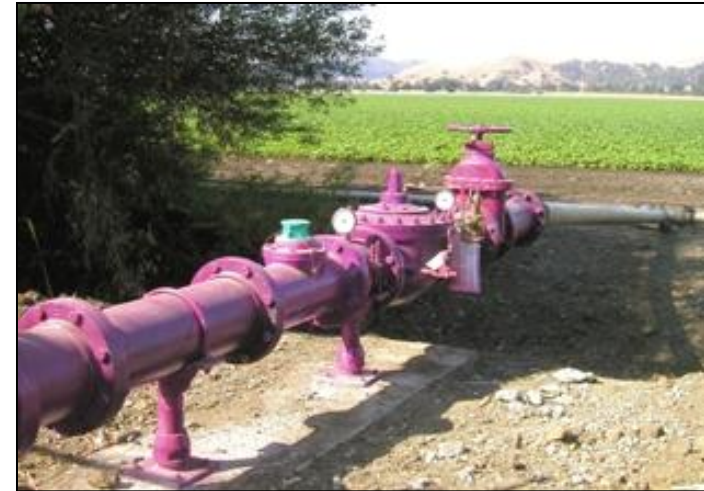
Purple lines to convey treated water
